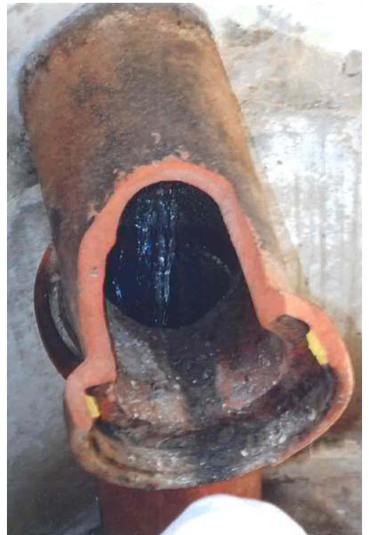
Photo #3: Canyon Springs - Joint Offset
