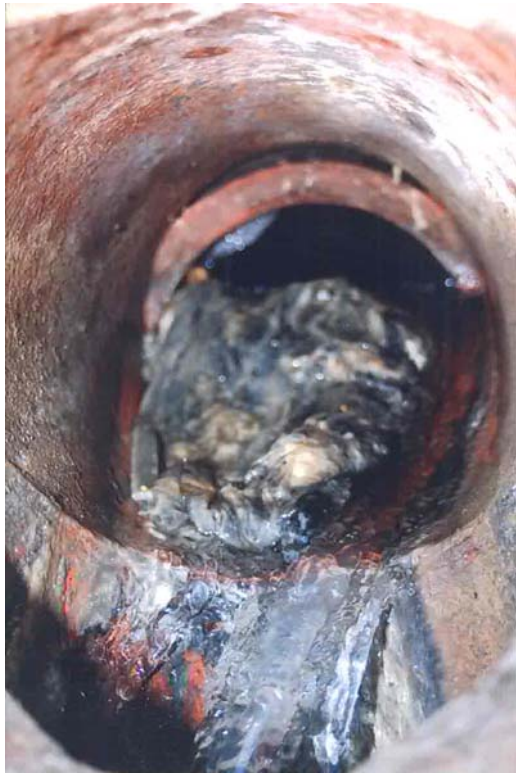
Photo #1: Canyon Springs - Joint Offset
