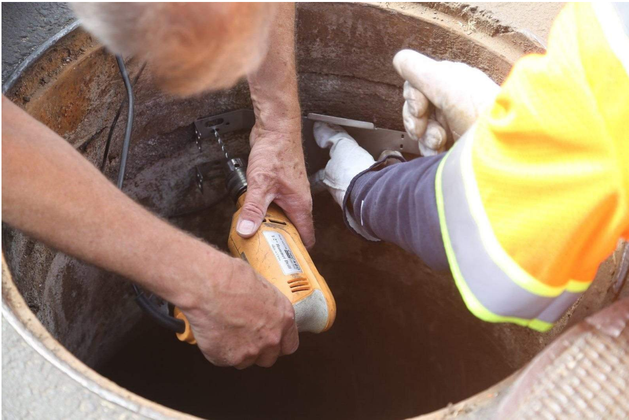
MANHOLE MONITORING SYSTEM INSTALLATION PHOTOS
