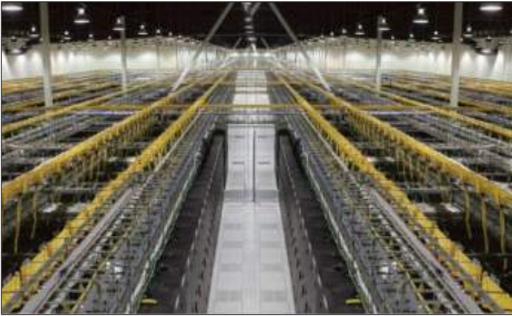
Mission operates its SCADA service from a carrier grade computer co-location center located near Atlanta, Georgia.
