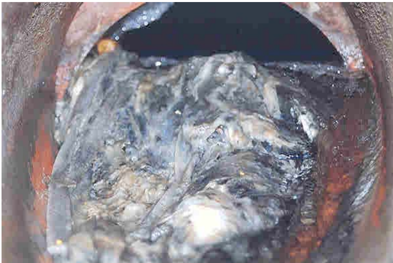
Photo #3: Canyon Springs - Joint Offset
