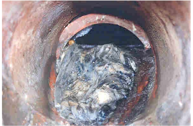
Photo #2: Canyon Springs - Joint Offset
