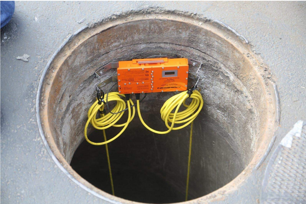
MANHOLE MONITORING SYSTEM INSTALLATION PHOTOS
